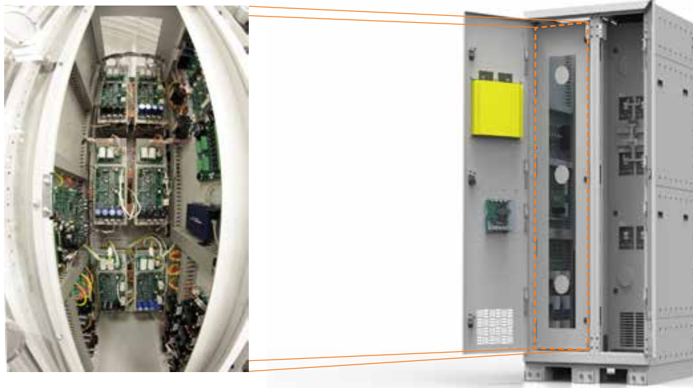
Polycarbonate Window on the Power Electronics Section, allowing visibility of status LEDs.
