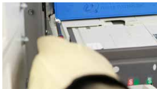
Screws Help Secure The Breaker
