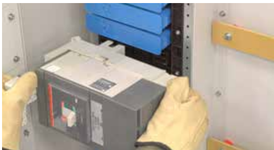
The Breaker Is Inserted Into The SafePanel
